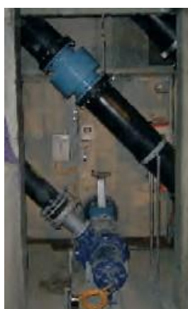
Pumpstation aus PE 100 Ø 200 ÷ 450
